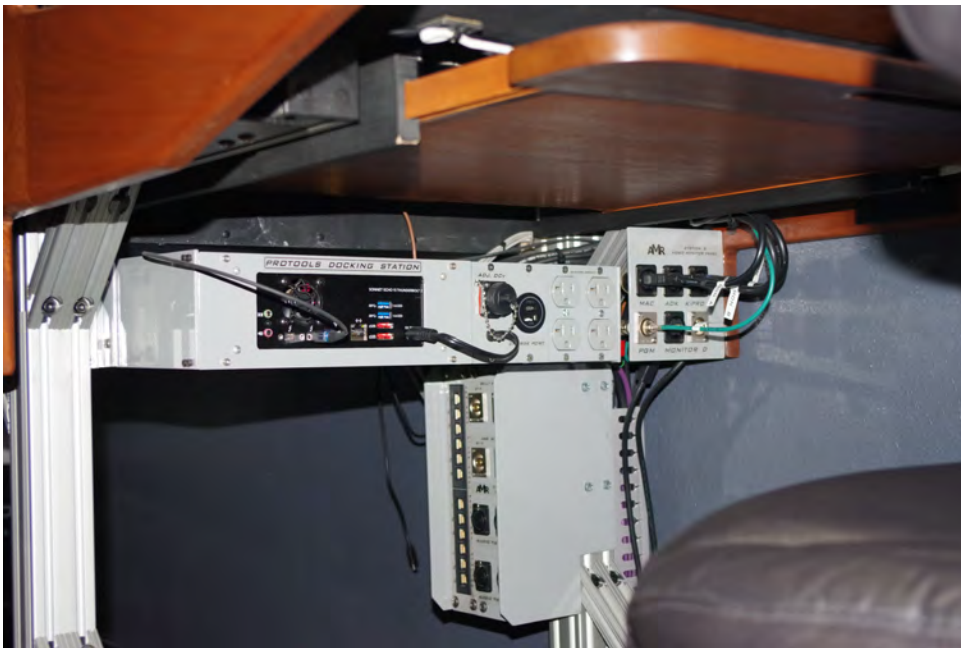
Local Thunderbolt Caddy with SSD Record Drives Audio, Video & Data Patch Lines
